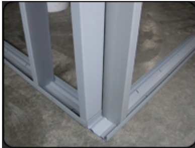
Add the next stud the same as you would if you creating an inside corner, this stud may be skipped if the inside corner will not have drywall on it
