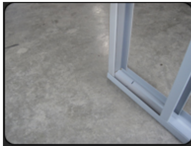
Assemble a wall with the end stud flush with the end of the track
